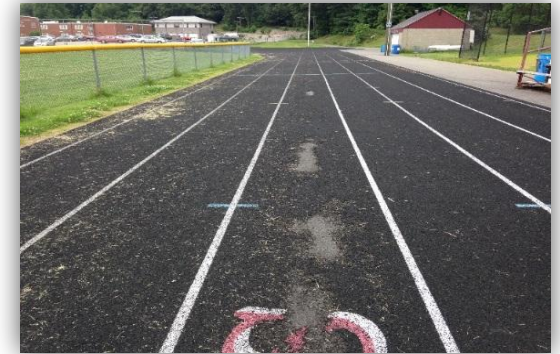
Worn Track Surfacing
