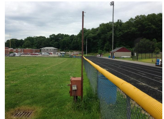
Electrical components outdated and misplaced
