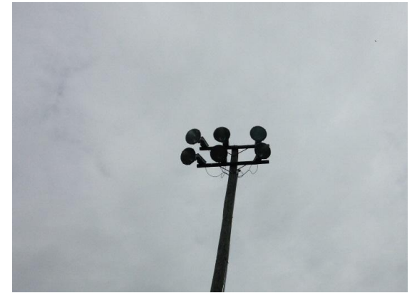
Existing light poles and balusters inadequate for multi-sport play
